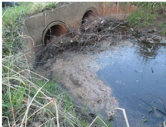
Photo 1. Naturally occurring foam at Nelson Bay Road drain, Williamtown. Photo: NSW EPA.
