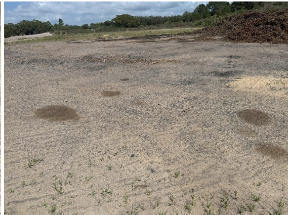
Photo 4: Minor hydrocarbon staining on truck parking area
